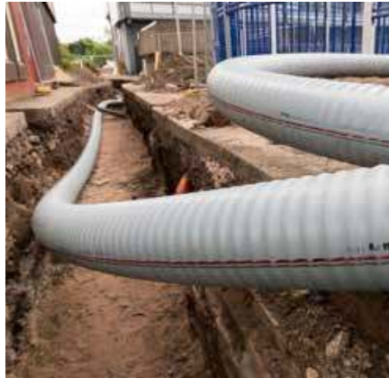
District heating & heat networks
